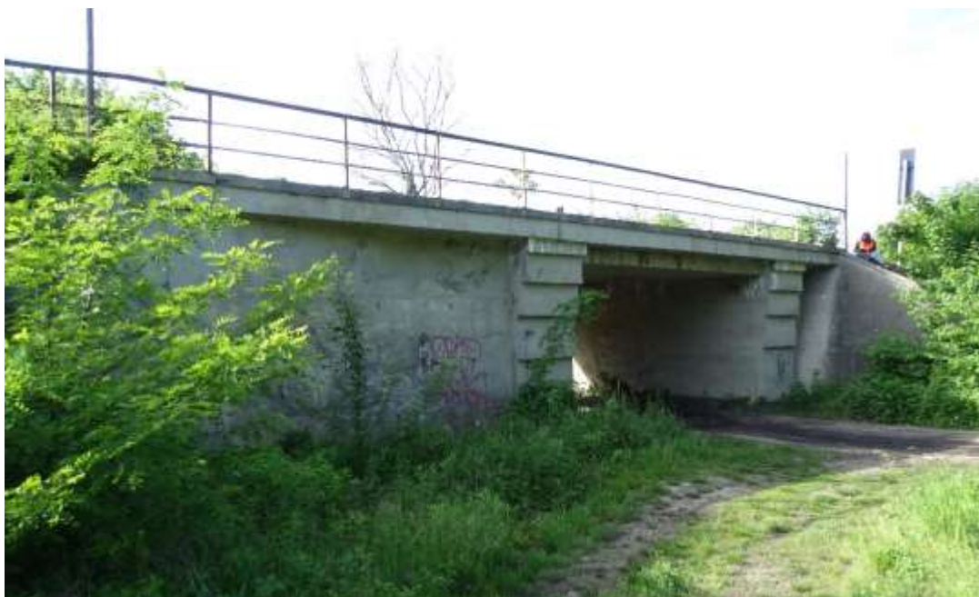
Fig. 2 View of the viaduct over Gorzyńska Street at 342,175 of the railway line No. 203
